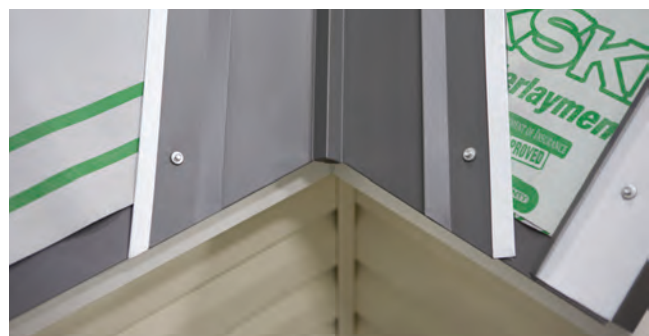
Fig. 16.4 - Anchor Cleat installed
