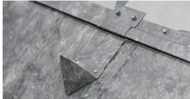
Fig. 39.1 - ProGrip diverter installed
