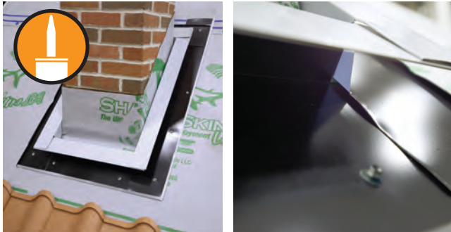
Fig. 25.2 - C-Closure installed with diverters
