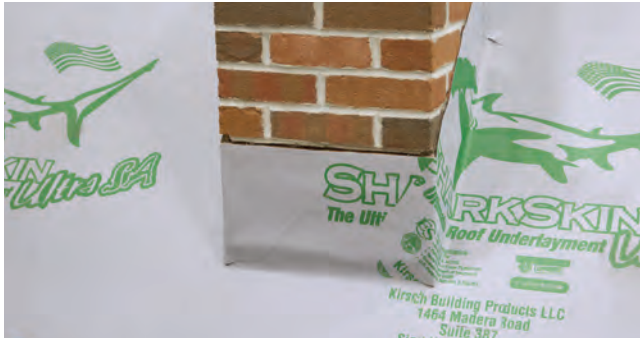
Fig. 25.1 - Chimney with 1" deep kerf
