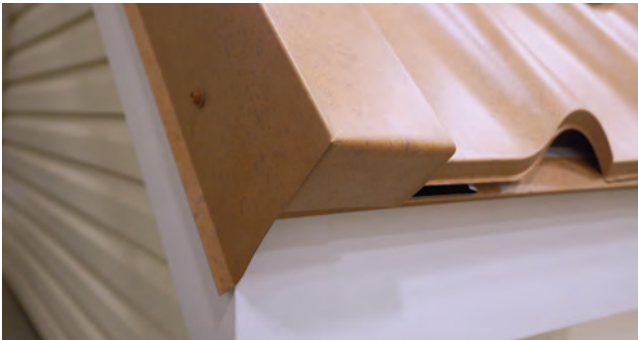
Fig. 13.1 - Rake installed over C-Closure
