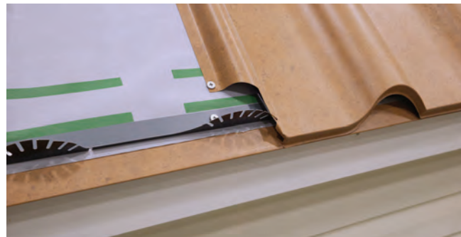
Fig. 18.2 - Bird Guard installed
